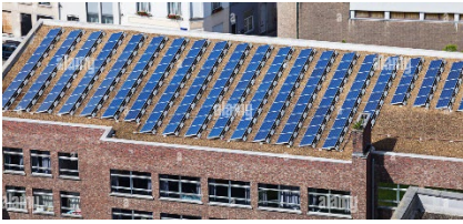
Solar Panels Roof Example
